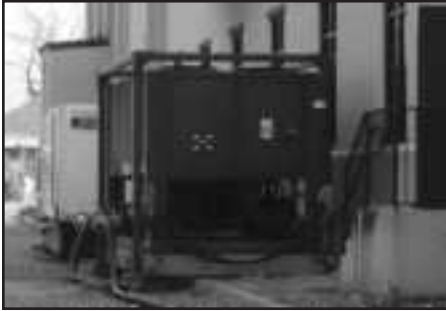
The generator outside the library. The generator helped regulate the temperature and humidity in the library. Photo by Karen Shaw.
